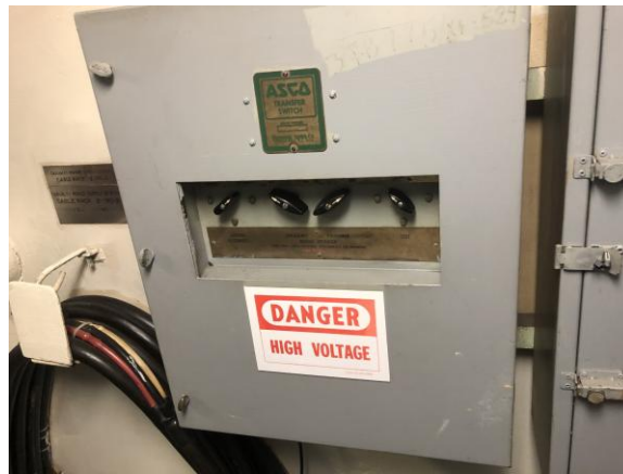
Figure 6: Automatic bus transfer on USS Midway (CV-41) (photos by Norbert Doerry)
