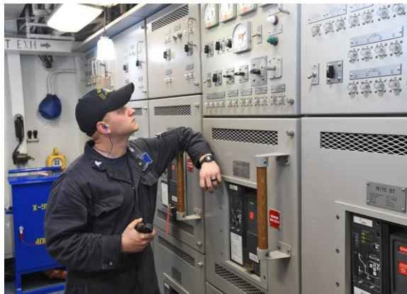
Figure 1: Switchboard on USS Blue Ridge (LCC 19) (US Navy photo)
