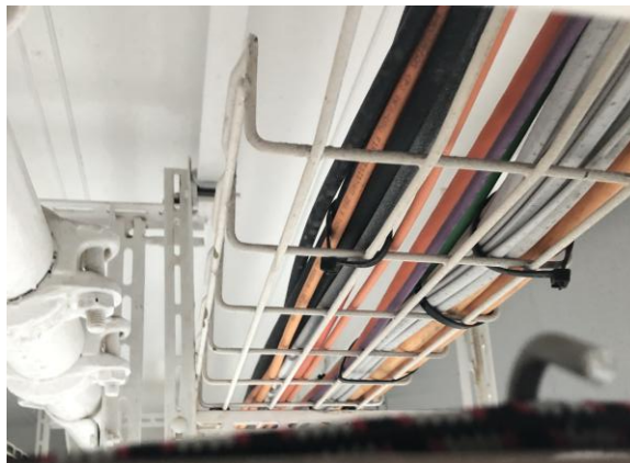
Figure 4: Electrical cables on Emerald Princess (photo by Norbert Doerry)
