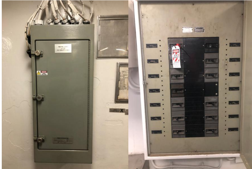
Figure 3: Power Panels on USS Wisconsin (BB 64) and N/S Savannah (photos by Norbert Doerry)
